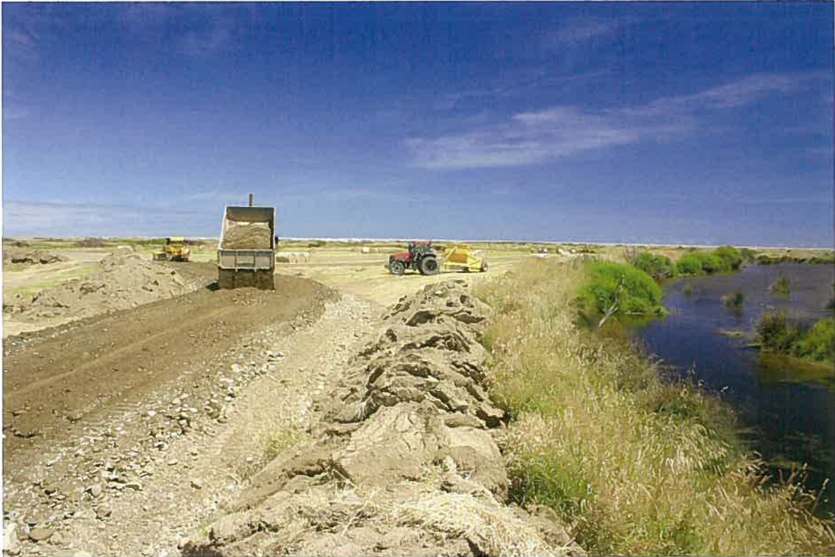
The Inder dam being built layer by layer, compacting the material with every pass of the machinery.
