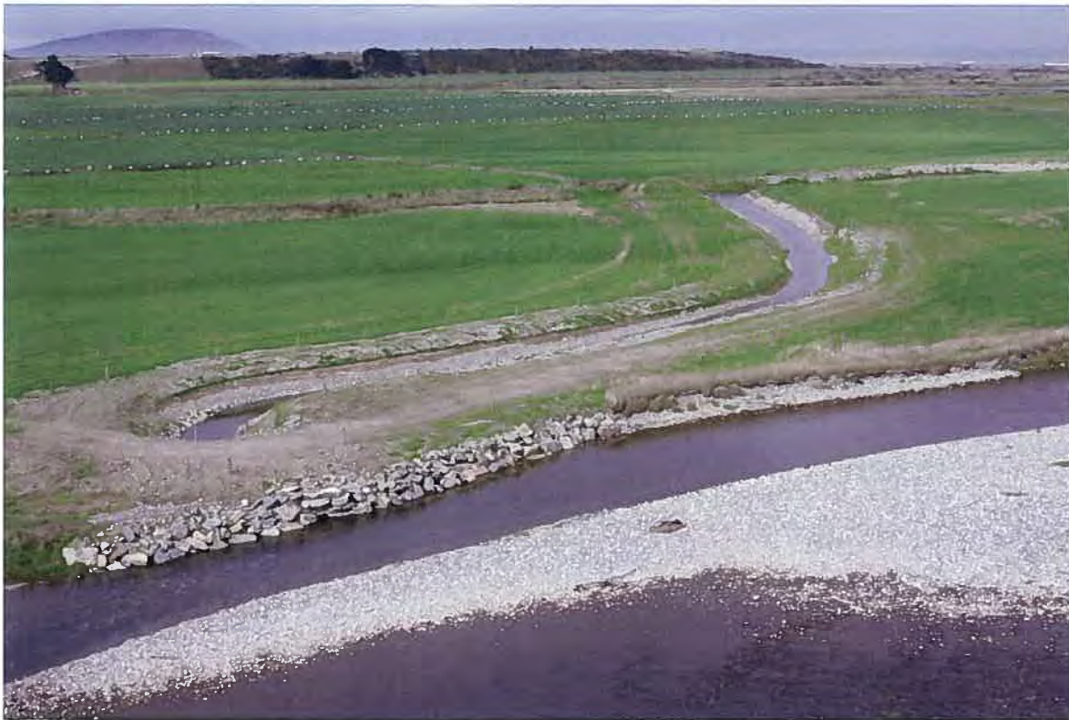
The completed diversion channel, showing the pipe intake, rock protection work and the Waiau River backwater from which the water is diverted for the Inder Wetland (Bill Jarvie April 2015).
