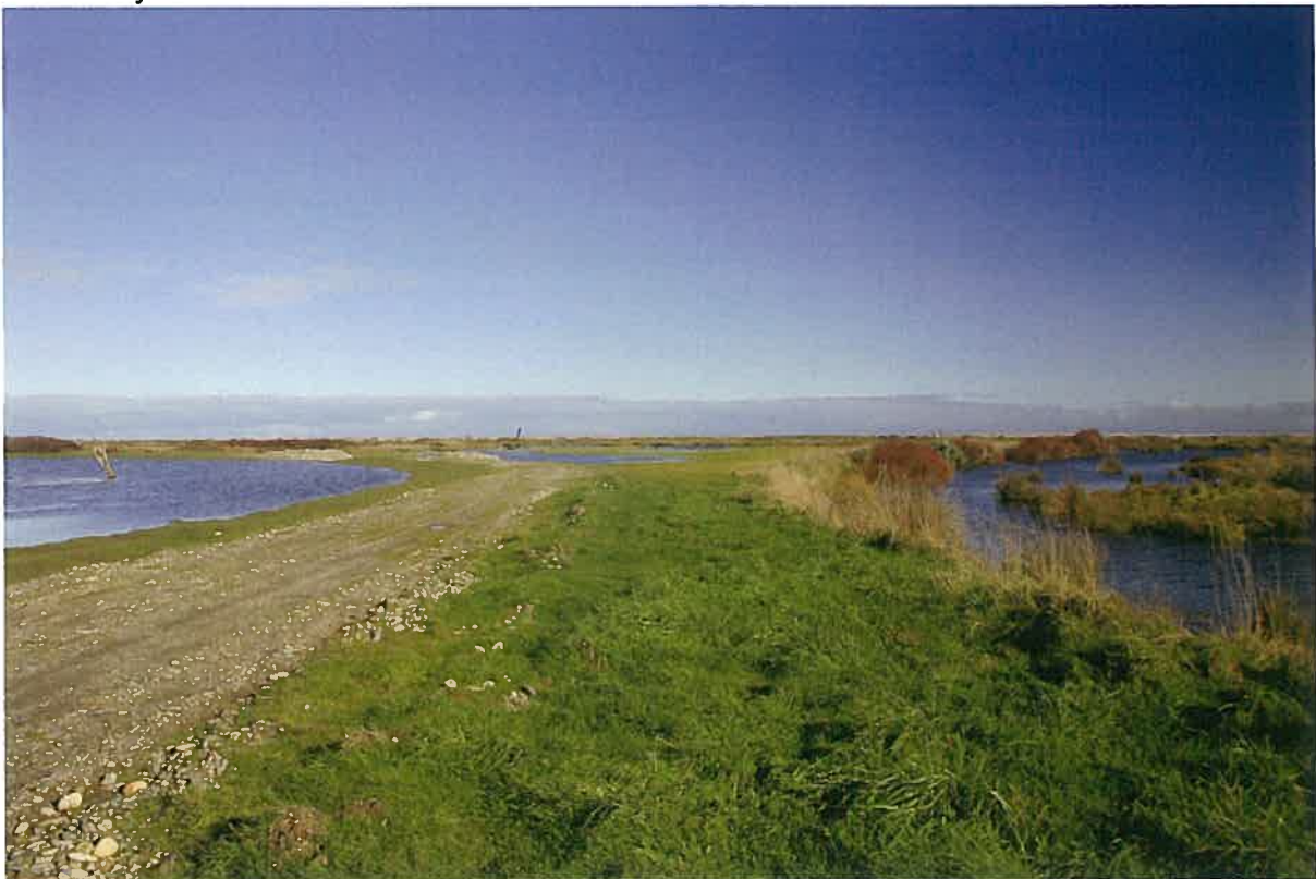
The completed dam. The existing McCulloch wetland is at the right of the photo. Water levels in this wetland are approximately 1 metre lower than in the Inder wetland.
