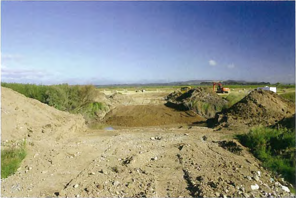
Site preparation and keying in the dam base through the zone of maximum height.
